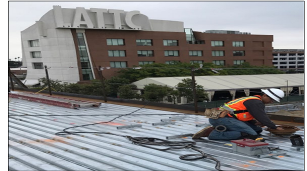
Anthony Montes- LATTC CMU Plumbing - Plumbers Local 78 Contractor: Pan Pacific Mechanical LA Trade Tech College - Culinary Arts Building
