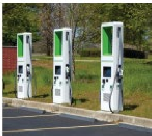
Electric vehicle charging
